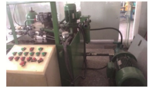
(b) Pump station
