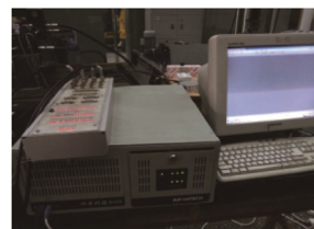
(a) dSPACE controller
