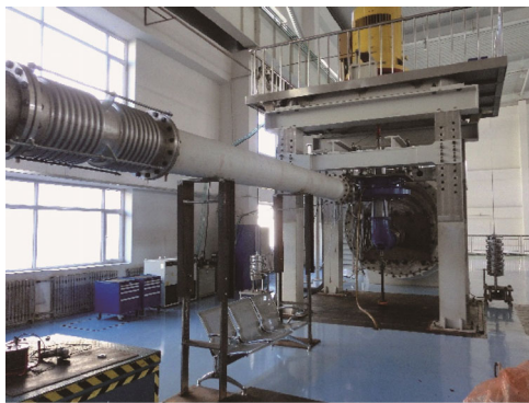
Fig. 1. Pump turbine model test rig installed at HEC, China
